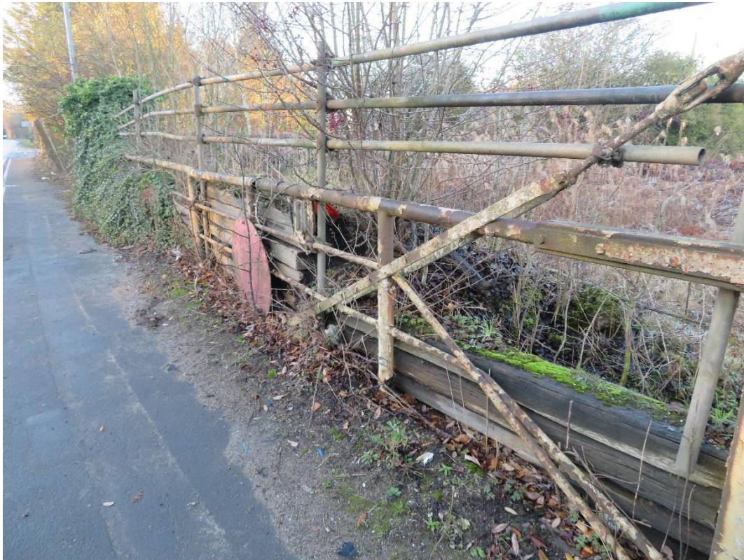
Plate 4 Part of the level crossing barriers towards Carrington Wharf on Manchester Road
